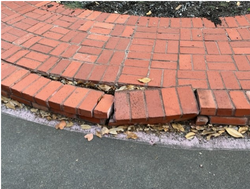
Brick Repairs needed at the Heard-Craig Center (Original brickwork done in the 1970s)
