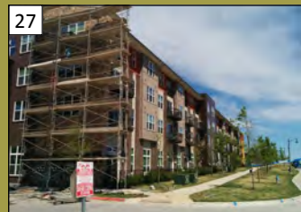
27 Parkside at Craig Ranch Phase II 7300 Henneman Way Valuation: $28.3 million Permit Issuance: December 2014
