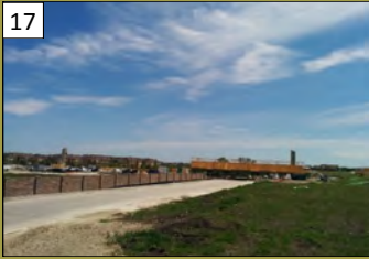
17 The Venue at Craig Ranch 4651 S. Custer Rd. Valuation: $21 million Permit Issuance: August 2015
