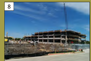
Parkside at Craig Ranch Phase III 6130 Alma Rd. Valuation: $48.4 million Permit Issuance: November 2015
