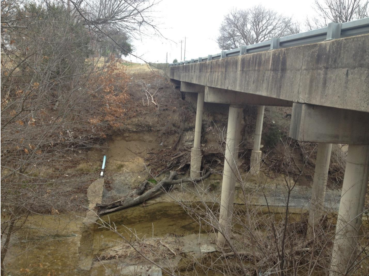
Custer Road bridge at Wilson Creek – shows incising of creek
