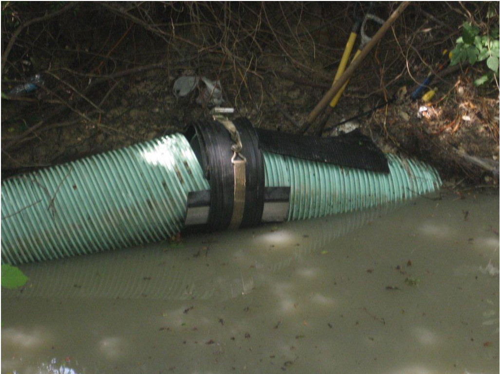
Sewer Break in Comegys Creek. Creek had eroded, exposing the pipe
