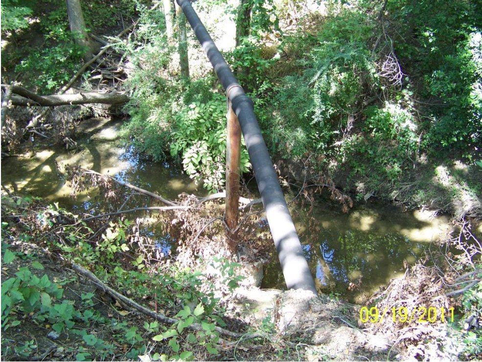
Jeans Creek Aerial Sewer Crossing impacted by creek scour
