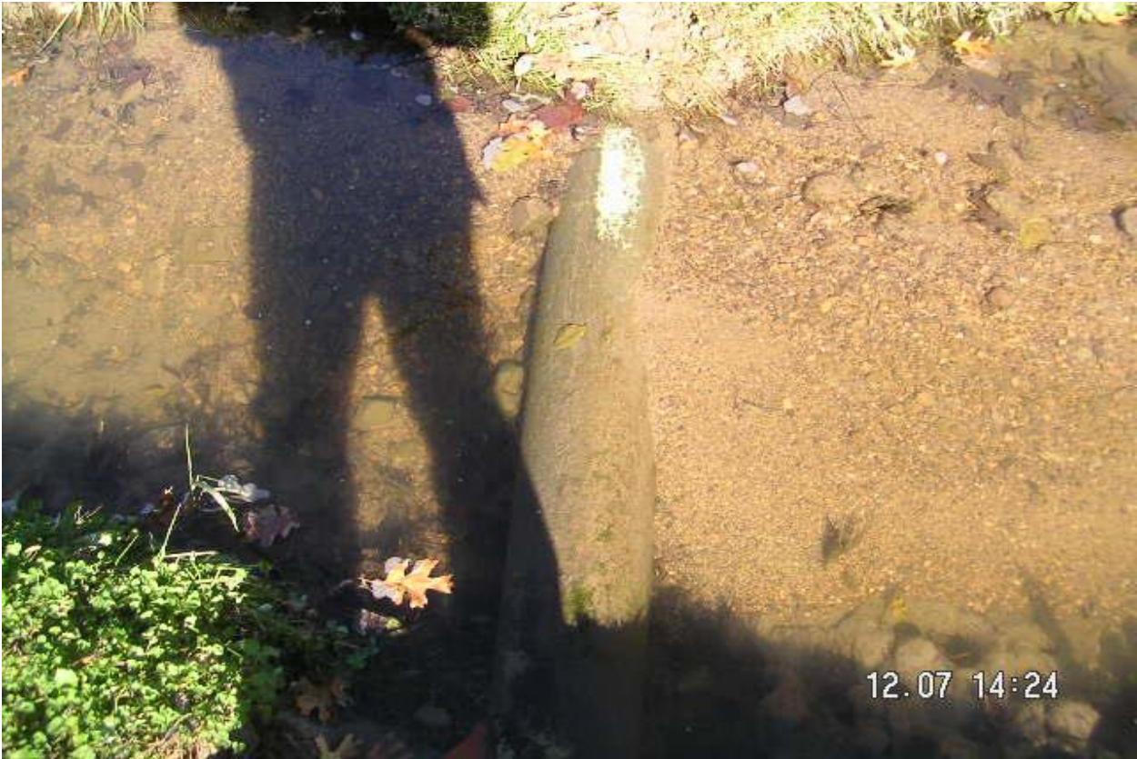
Finch Park exposed sanitary sewer
