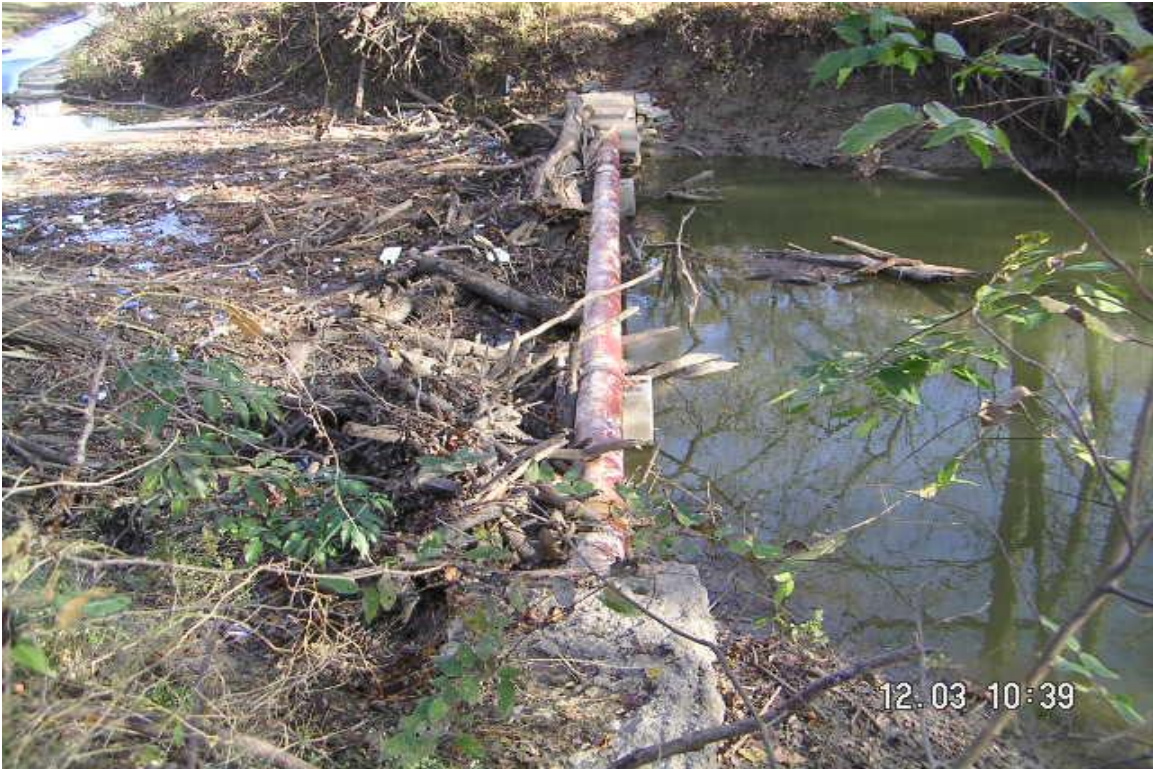
Aerial sewer crossings catching debris
