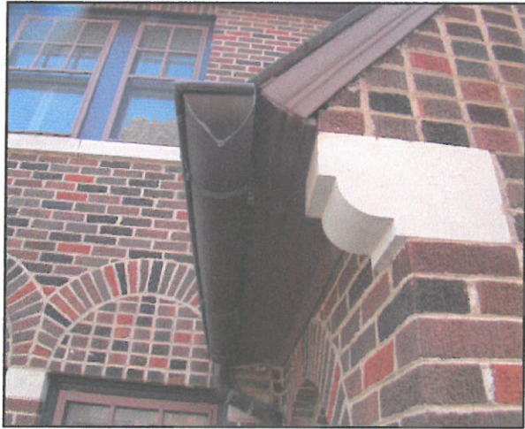
Newly developed "carpet" brick by Acme in 1924 is laid in varied courses.
