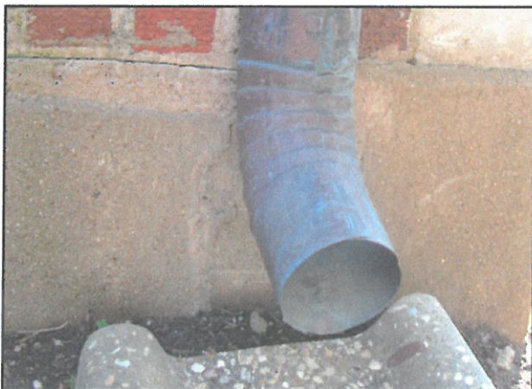
The original drainage system made of copper is in excellent condition.
