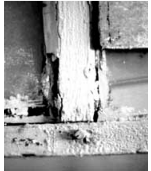
This historic double-hung window has many layers of paint, some cracked and missing putty, slight separation at the joints, broken sash cords, and one cracked pane. Photo: NPS files.
