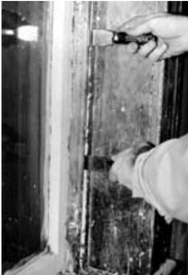
After removing paint from the seam between the interior stop and the jamb, the stop can be pried out and gradually worked loose using a pair of putty knives as shown. Photo: NPS files.
