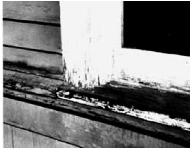
Deterioration of poorly maintained windows usually begins on horizontal surfaces and at joints, where water can collect and saturate the wood. Photo: NPS files.
