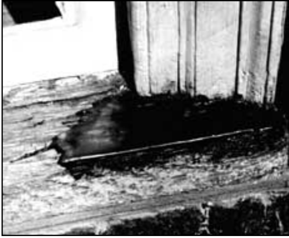
This illustrates a two-part epoxy patching compound used to fill the surface of a weathered sill and rebuild the missing edge. When the epoxy cures, it can be sanded smooth and painted to achieve a durable and waterproof repair. Photo: NPS files.
