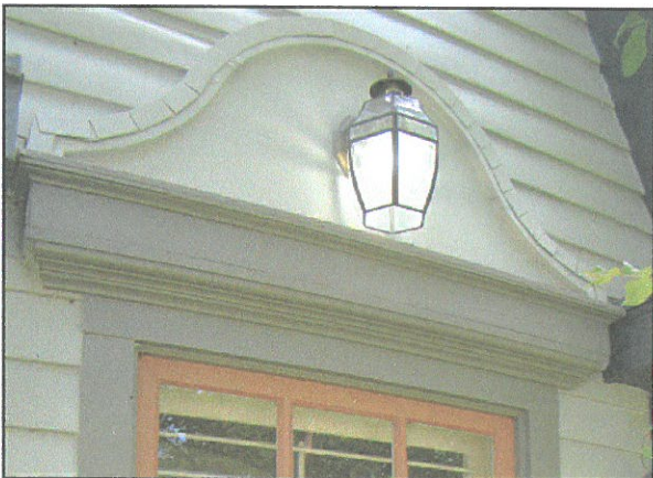
The bell arch over the front window adds to the upward thrust of the spire-like gable.
