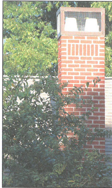
Builder J. Ed Michael added a "soldier course" as a chimney detail.
