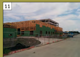
11 Parkside at Craig Ranch Phase III 6130 Alma Rd. Valuation: $48.4 million Permit Issuance: November 2015
