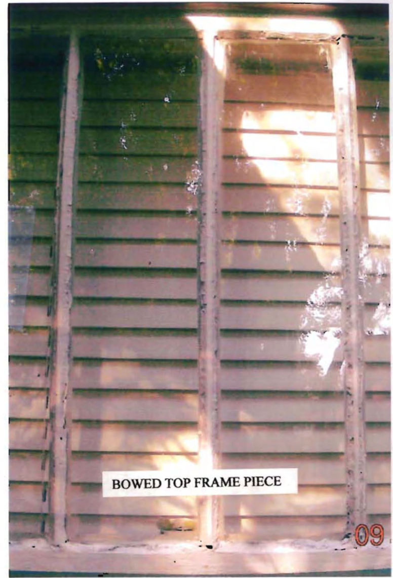
DETERIORATION OF GLAZING AND PAINT
