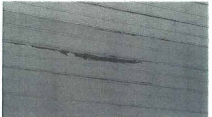
Ceiling damage from faulty roof
