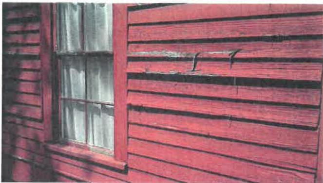
Peeling exterior paint
