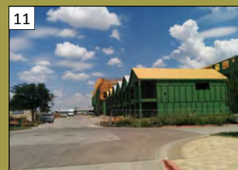
Parkside at Craig Ranch Phase III 6130 Alma Rd. Valuation: $48.4 million Permit Issuance: November 2015
