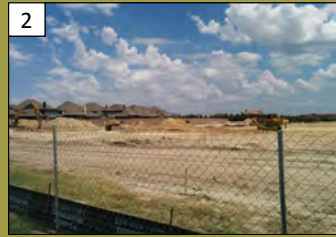
Artistry Senior Residence at Craig Ranch 8950 Collin McKinney Pkwy. Valuation: $20 million Permit Issuance: June 2016
