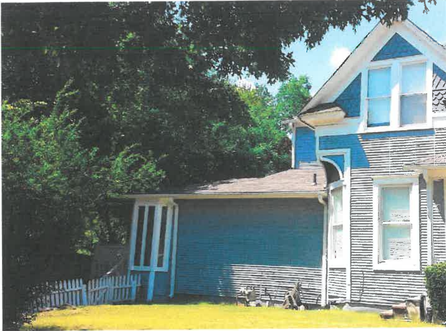
Current addition – view 1 - Roofline, windows, & trim do not match the character of the original (2 story) home.
