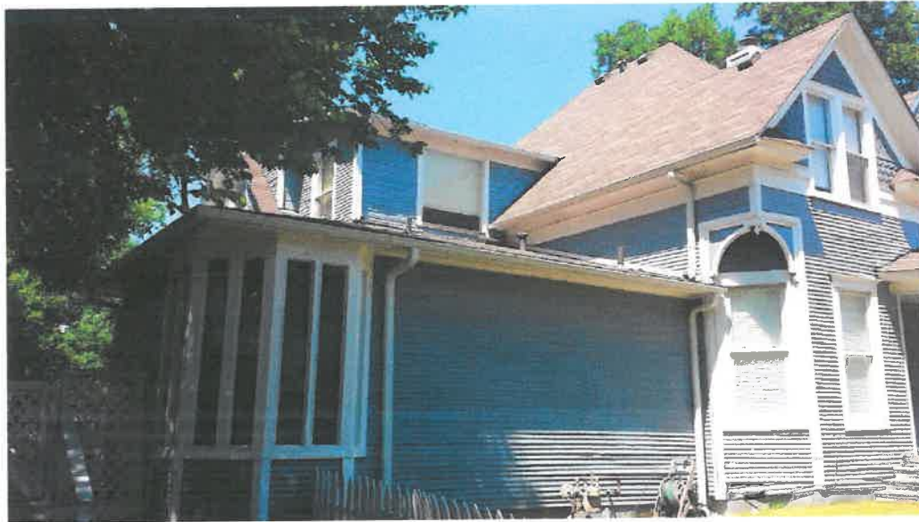
Current addition – view 2 - Roofline, windows, & trim do not match the character of the original (2 story) home.
