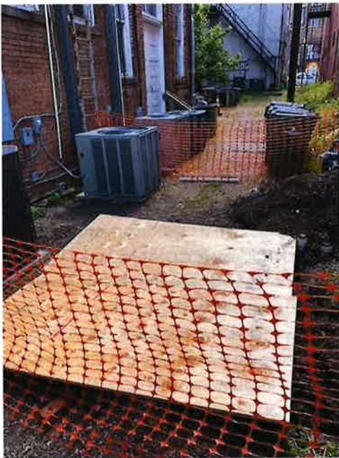
EXCAVATED GREASE TRAP REMOVED FROM THE GROUND AND ABANDONED BY JASON BRIDSCHGE, OWNER TCB CONTRACTOS
