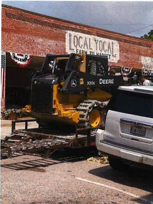
SKID STEER USED TO DELIVER GREASE TRAP SECOND TIME DRIVEN BY PRECON PRECAST LLC EMPLOYEE. DROVE OVER/CRUSHED CITY WATER LINES IN DOWNTOWN MCKINNEY.
