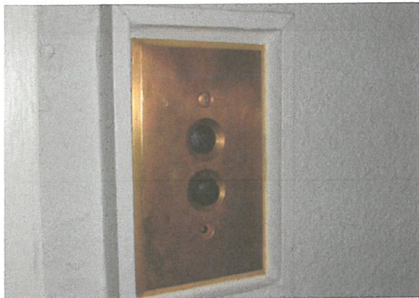
Brass switch plate is framed by molding.
