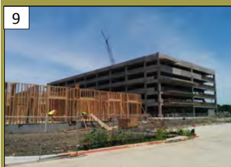
9 Parkside at Craig Ranch Phase III 6130 Alma Rd. Valuation: $48.4 million Permit Issuance: November 2015
