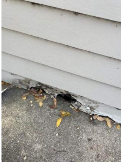
705 N College St #2 (Siding Damage)
