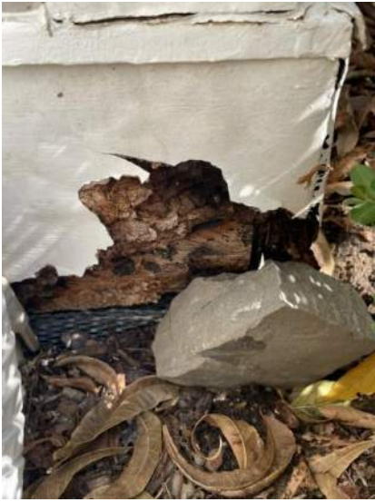
705 N College St #1 (Trim Damage)
