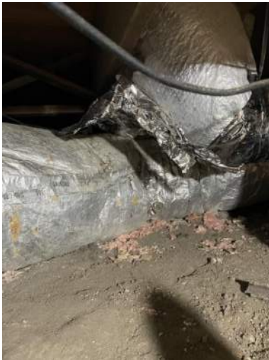
705 N College St #4 (HVAC Issue).
