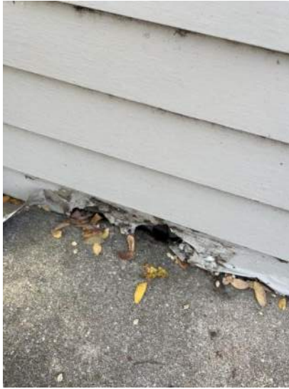
705 N College St #2 (Siding Damage)
