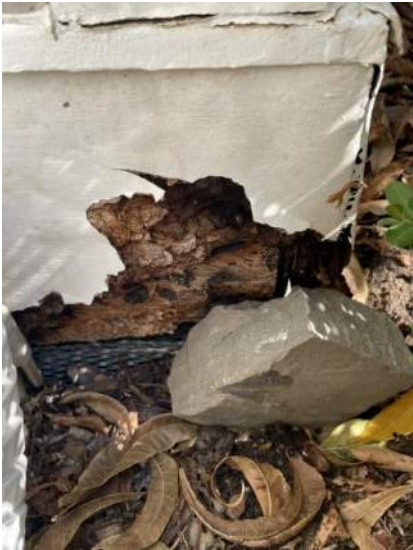
705 N College St #1 (Trim Damage)
