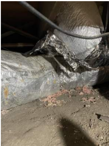
705 N College St #4 (HVAC Issue).
