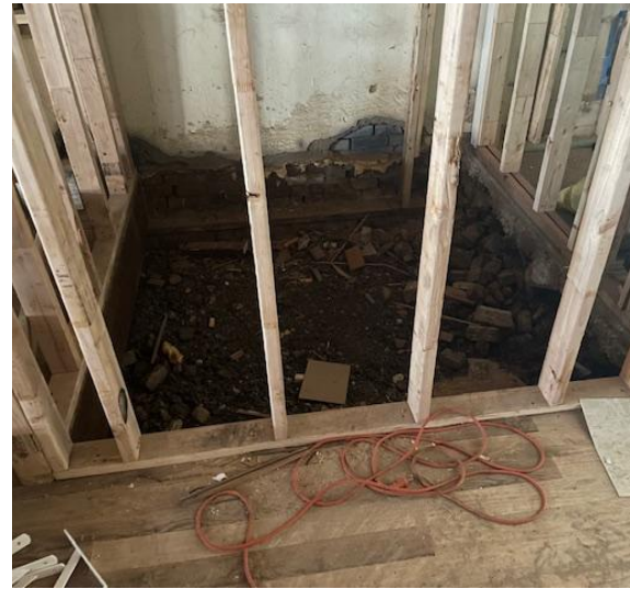
Current Grease Trap Plan in Progress
