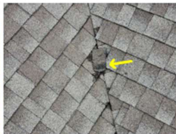
Shingle damage (possible source of water stain in southeast office ceiling)
