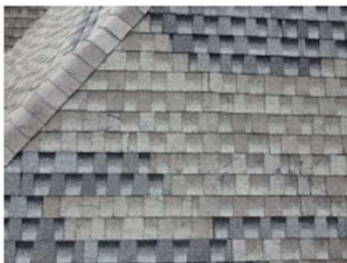
Previous repairs to roofing materials
