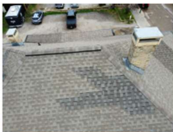
Previous repairs to roofing materials
