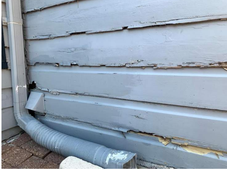
Left: condition of removed siding Middle: bay window during rehabilitation Right: condition of siding pre-removal
