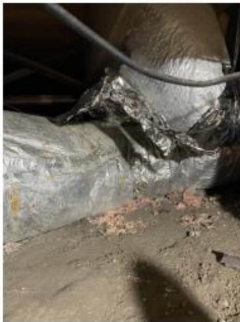
705 N College St #4 (HVAC Issue).
