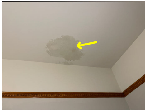
Upstairs south east office: water stains
