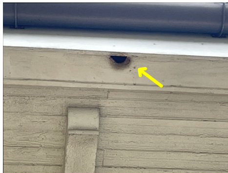
Front exterior soffit: Rodent damage/entry point
