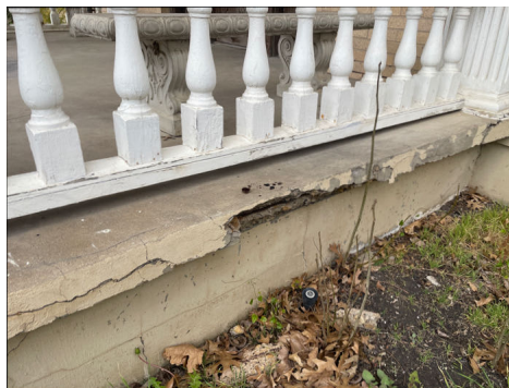
Front Porch Damage
