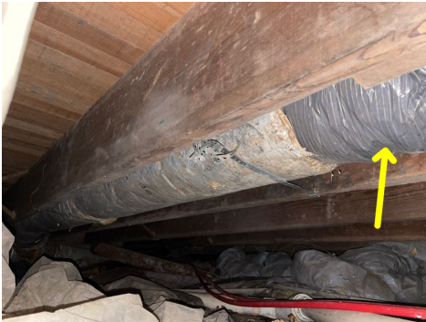
Crawlspace: Flex duct in crawlspace
