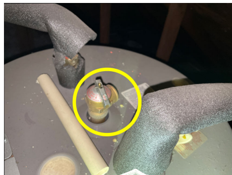
Attic: TPR discharge line missing
