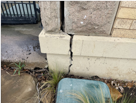
Foundation corner damage
