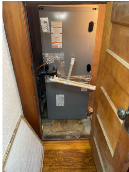
Downstairs System: HVAC
