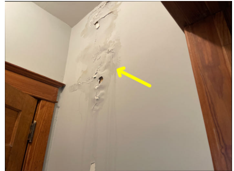
Upstairs south of office: Water damage
