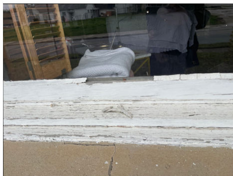
Window paint, caulk, and glazing deterioration
