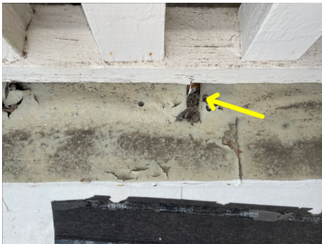
Front porch peeling paint
