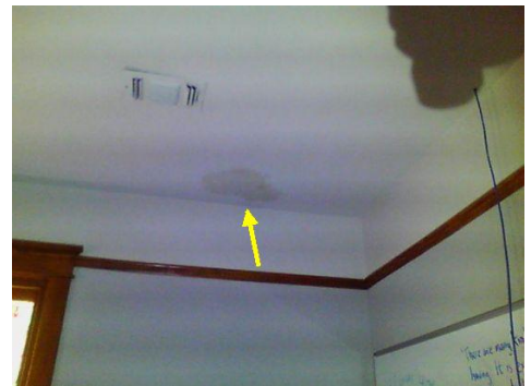
Upstairs southeast office: water stain
