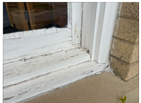
Window paint, caulk, and glazing deterioration
