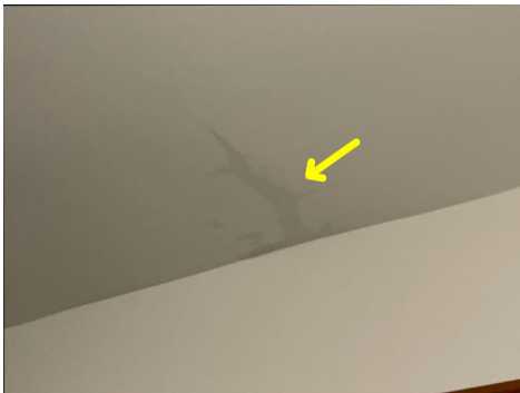
Upstairs Hall: Ceiling Water Stains
