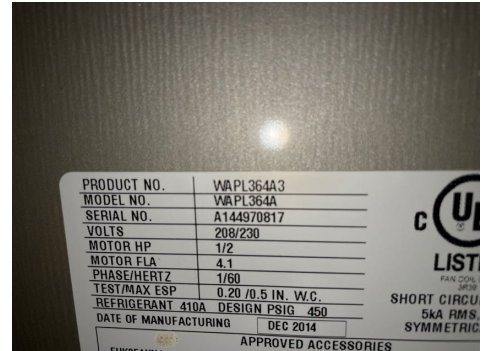
Upstairs South System: Furnace Label
