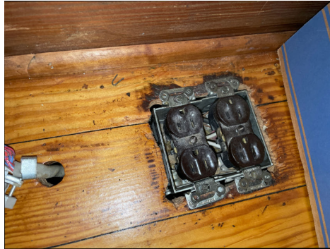
Upstairs NE corner: Floor outlet missing cover
