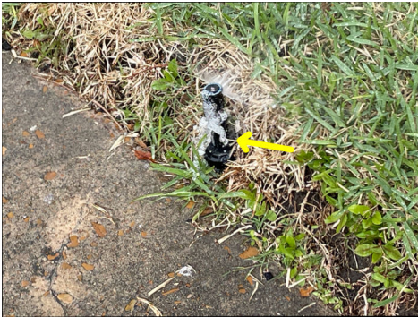
Sprinkler head damage
