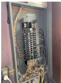
Sub Panel with front removed
