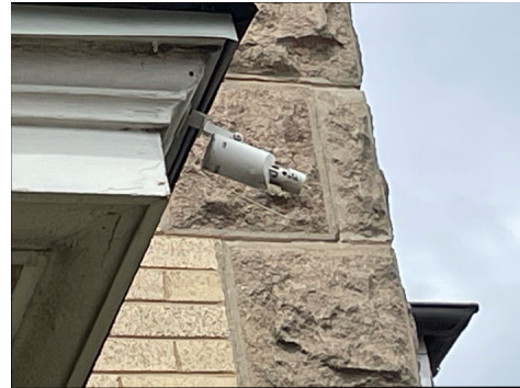
Rain Sensor Not Installed Vertical
