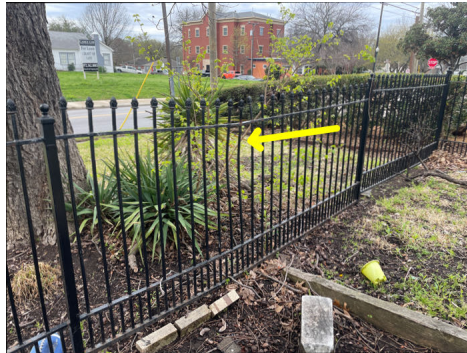
Minor fence damage
