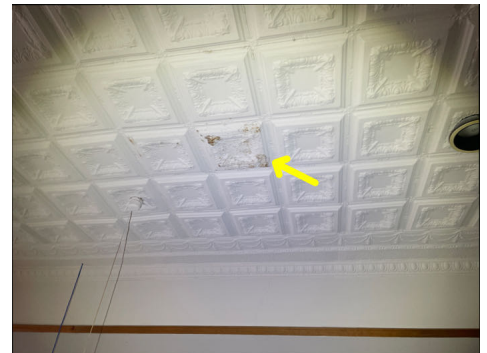
Upstairs North Office: Ceiling Water Stains
