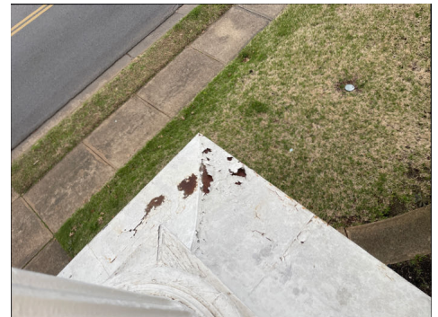
Front porch peeling paint
