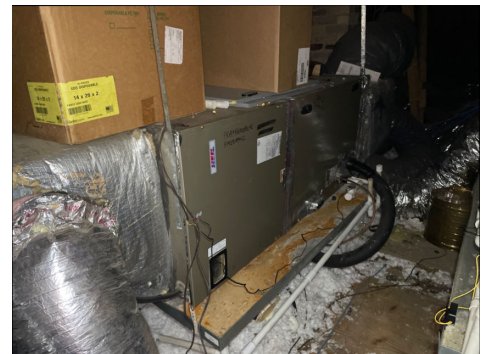
Upstairs NE Corner: HVAC unit in attic
