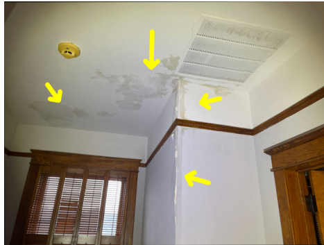
Top of west stairs: Water damage
