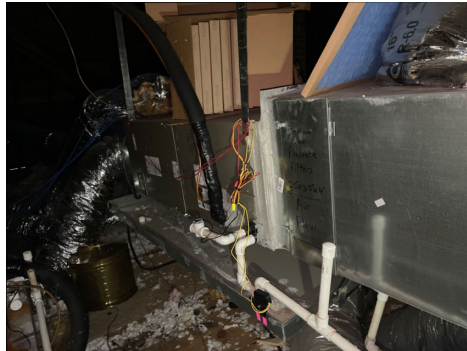
Upstairs South System: HVAC unit in attic
