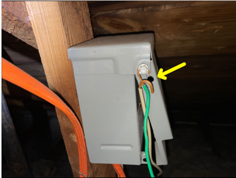
Attic water heater: Loose/improper grounds
