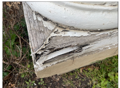
Front Porch Damage
