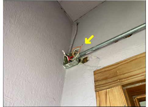
Downstairs Suite 132 Closet: Connection not in Junction Box
