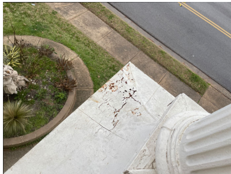
Front porch peeling paint
