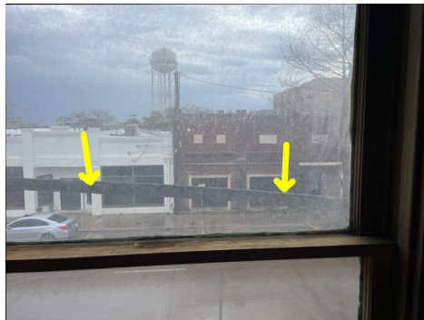
East exterior: Service wires are too close to window openings
