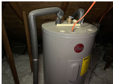
Attic: Water Heater
