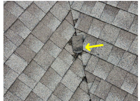
Shingle damage (possible source of water stain in southeast office ceiling)
