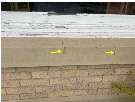
Exterior window sill damage
