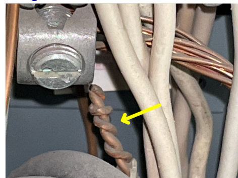
Sub Panel: neutral connection missing wire nut
