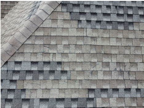
Previous repairs to roofing materials
