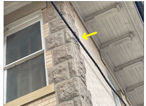
East exterior: service wires too close
