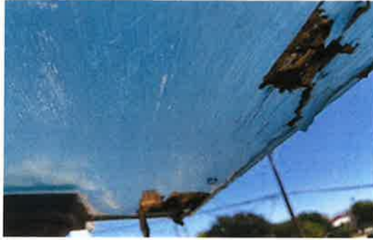
Unsupported existing covered porch
