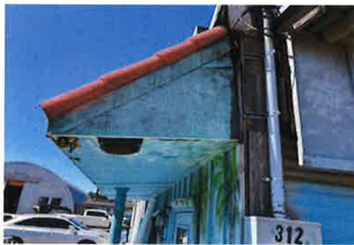
Missing column leaning covered porch area before Existing metal siding with rotten wood replaced
