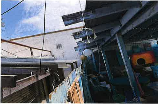
Existing rear fence and Rotten wood from patio cover rafters
