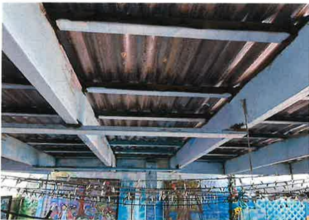
Rotten painted wood on rafters and rear fence
