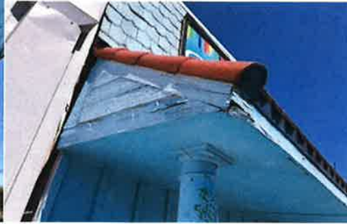
Existing covered porch area rotten wood siding
