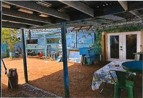
Existing patio cover double sloped to center Rotten wood
