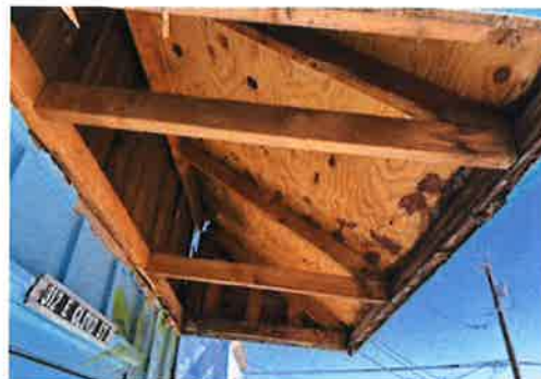
Rotten wood framing/structure
