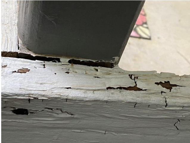
All photos from 2023 showing condition of home before rehabilitation project
