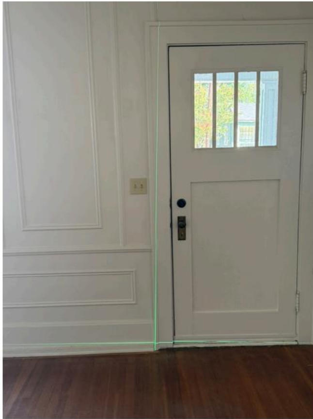
Above: Walls out of plumb.
