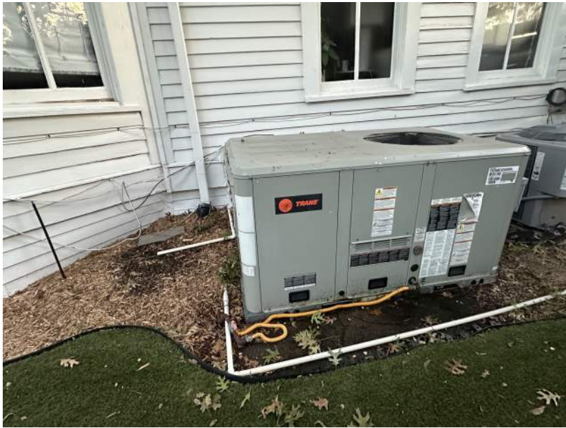
EXISTING 4T PACKAGE UNIT THAT IS TO BE REPLACED
