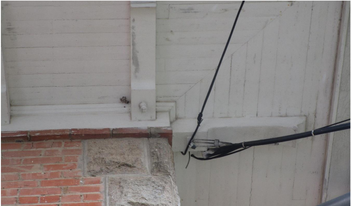
Photo #5 Close up of roof soffit at the northwest corner of building. The utility lines do not appear to have damaged the soffit structure.
