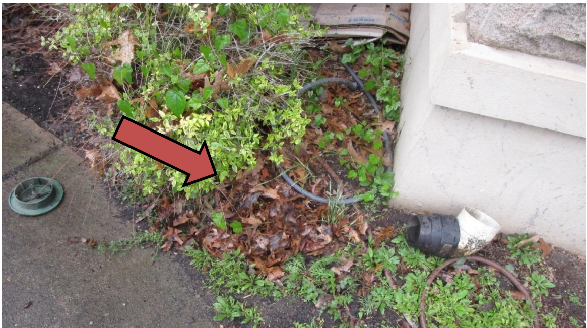
Photo #16 Arrow points to debris covered exit for the pipe that is connected to the downspout. No water is flowing out from the pipe shortly after a rain event. This should be tied to an underground drain that discharges at the curb.
