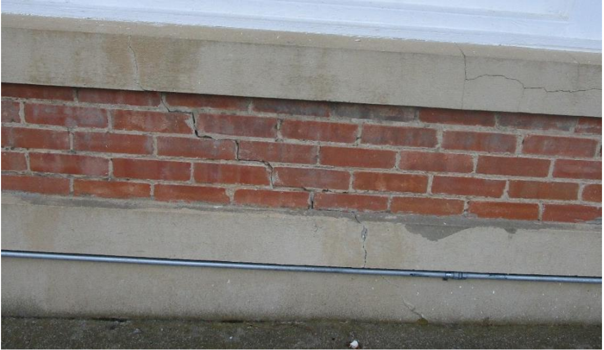
Photo #63 Crack in the brick and foundation under the window on the north side of the building.
