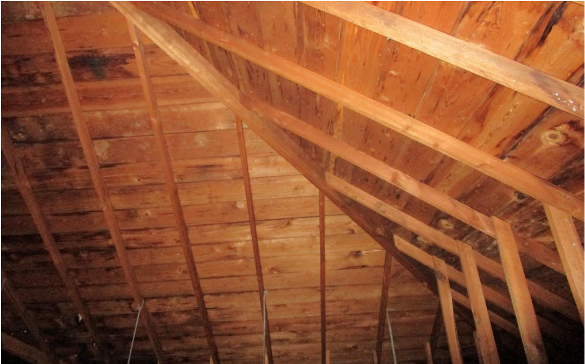
Photo #47 Southwest corner of the roof. Some water staining is visible on the roof deck on the left side of the photo.
