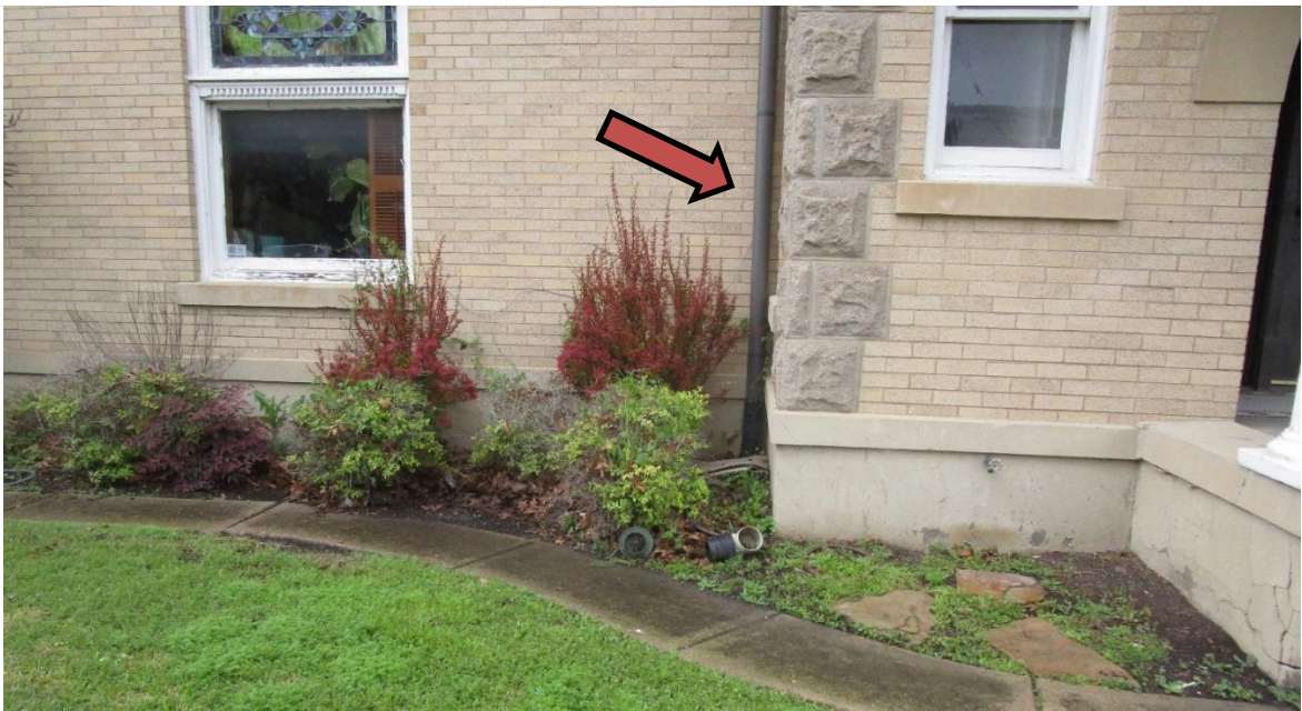
Photo #14 Yard area just south of the east entrance covered porch. The arrow points to a downspout nestled in the corner. This should be tied to an underground drain that discharges at the curb.
