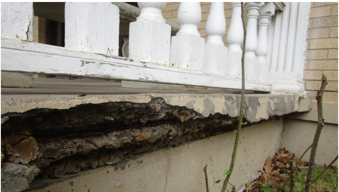
Photo #20 Close up of severely rusted rebar on the east side of the covered patio.
