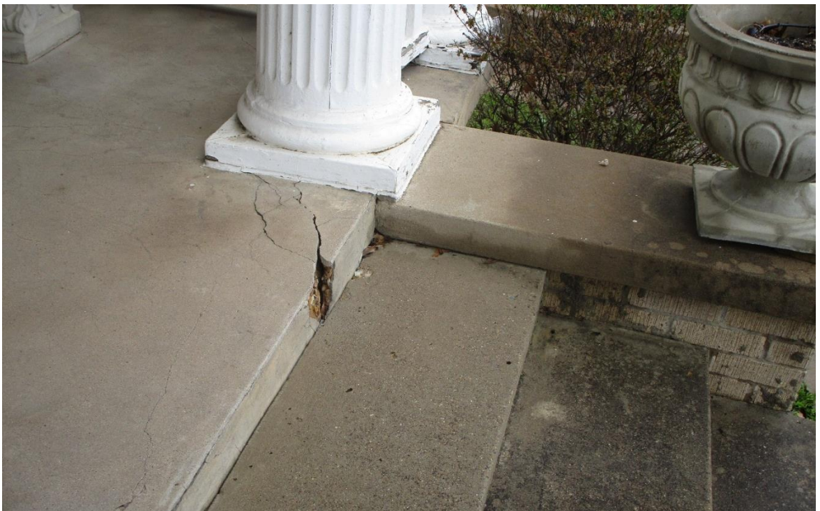
Photo #28 Damaged concrete slab at the south patio.
