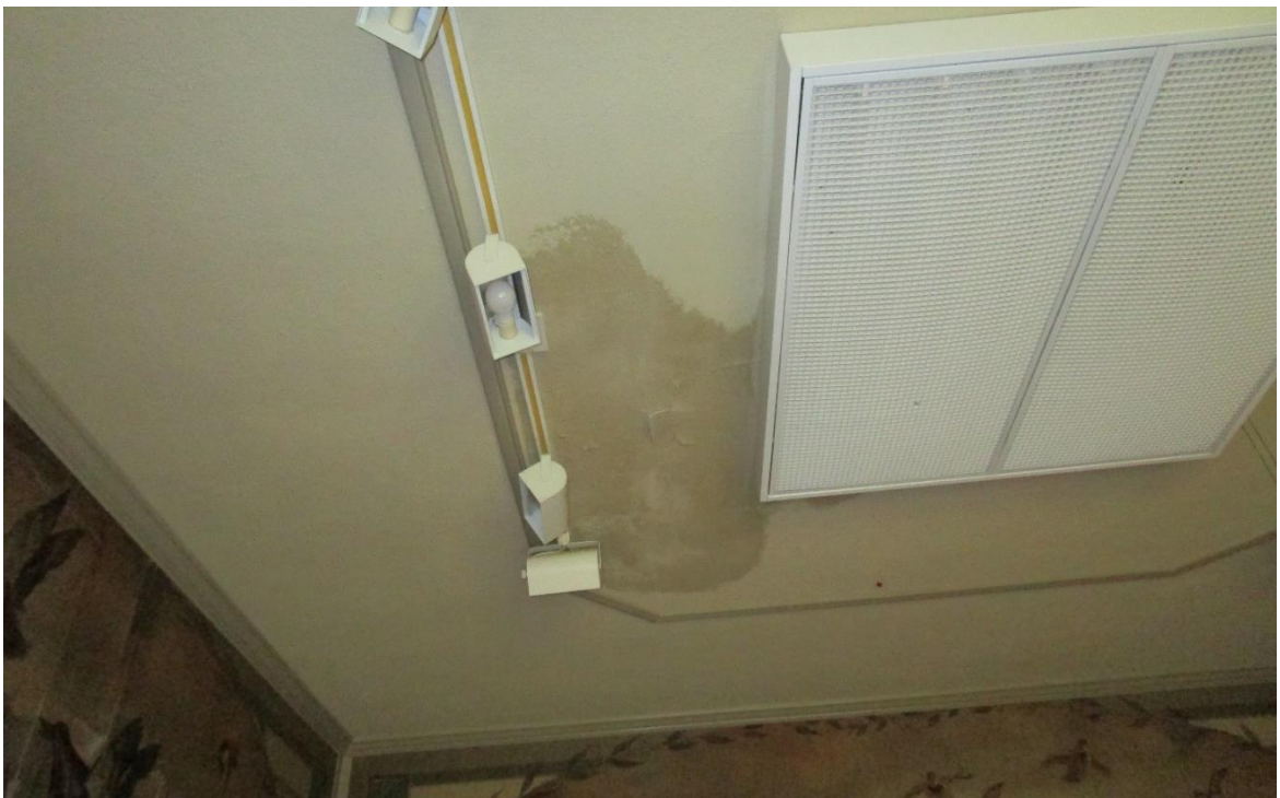
Photo #36 Water damage to a ceiling on the first floor.
