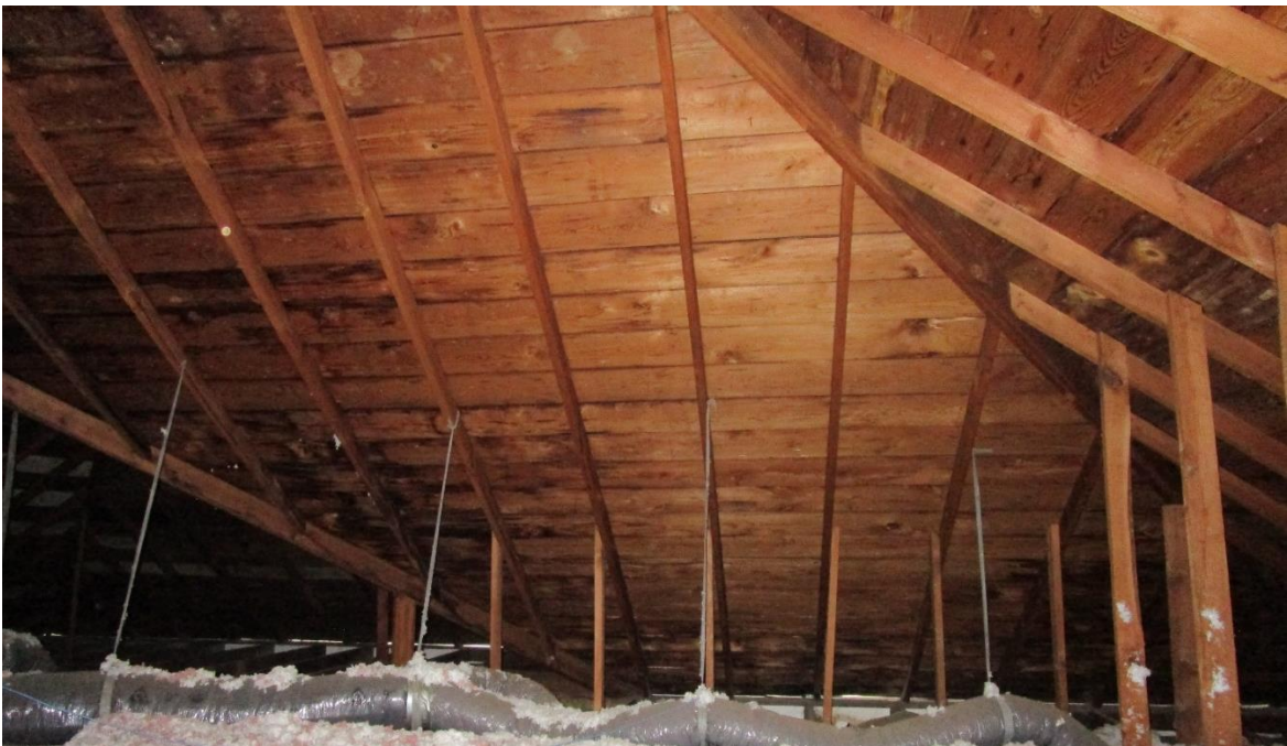
Photo #46 Underside of the west portion of the roof. The roof rafters are 2x4's at 24 inches on center and are spanning way beyond the code allowable spans. The decking on the left side of the photo has a lot of water staining.
