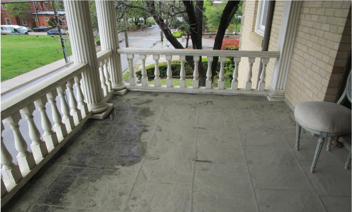
Photo #49 View of second floor balcony above the south entrance. The floor appears to be soldered tin.
