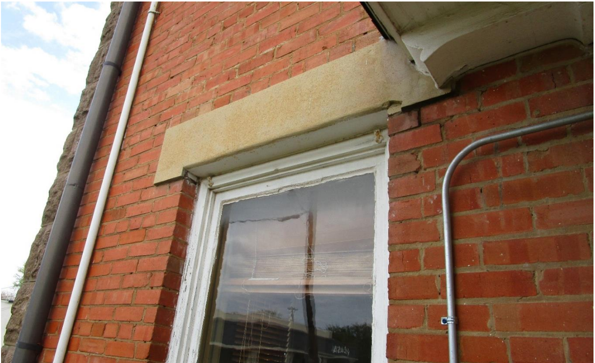
Photo #60 Window on the west side of the building has some water damage at the upper right-hand corner
