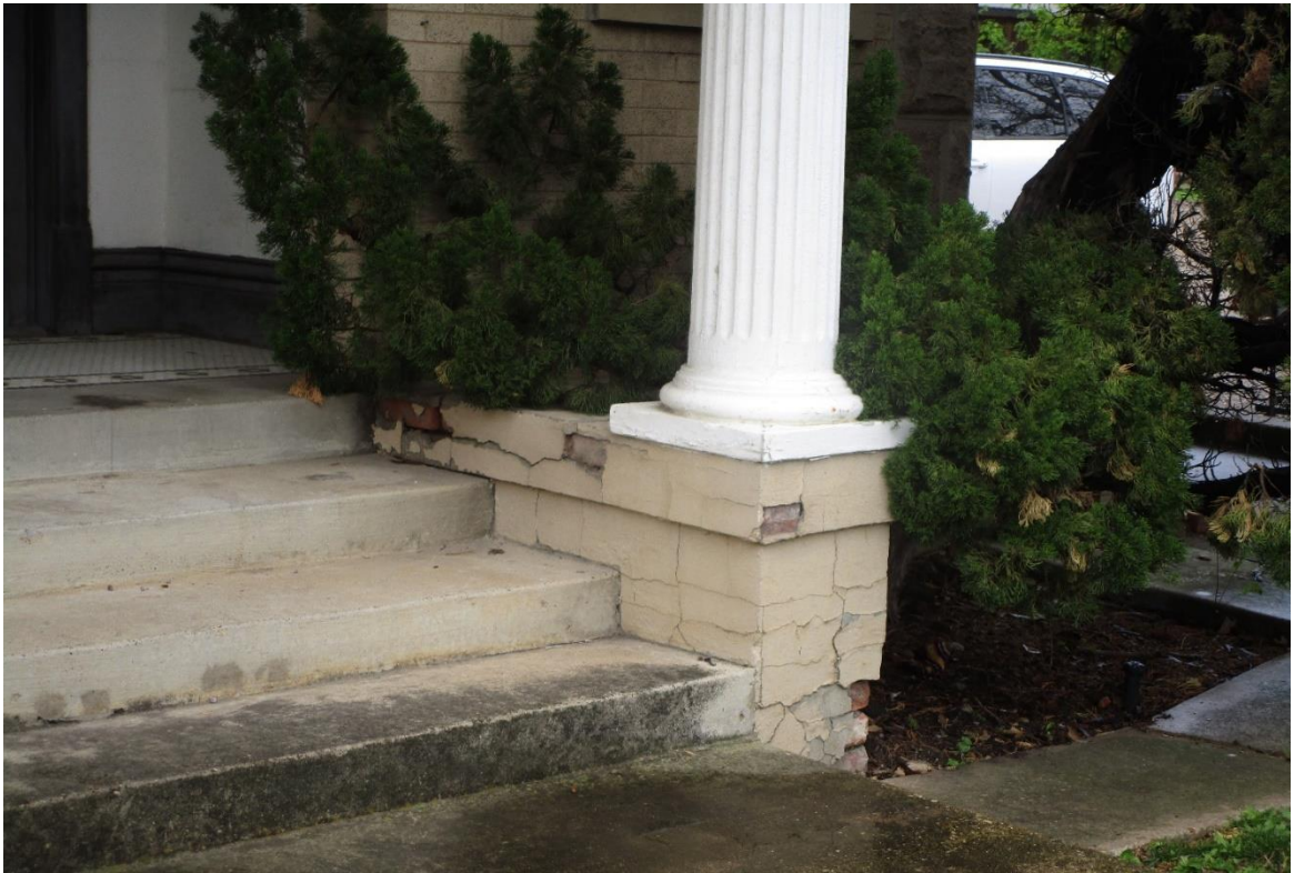
Photo #13 Another view of the damaged brick wall on the north side of the covered porch entrance.
