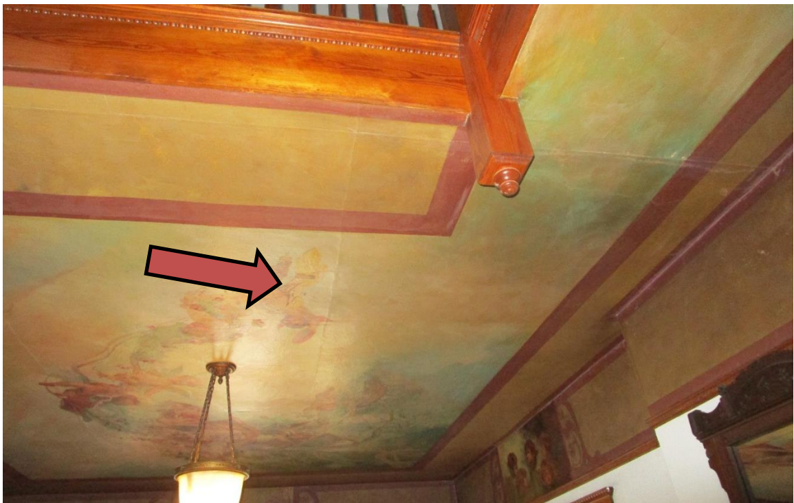
Photo #38 The arrow points to a crack in the ceiling mural. The crack is likely due to water from a roof leak.
