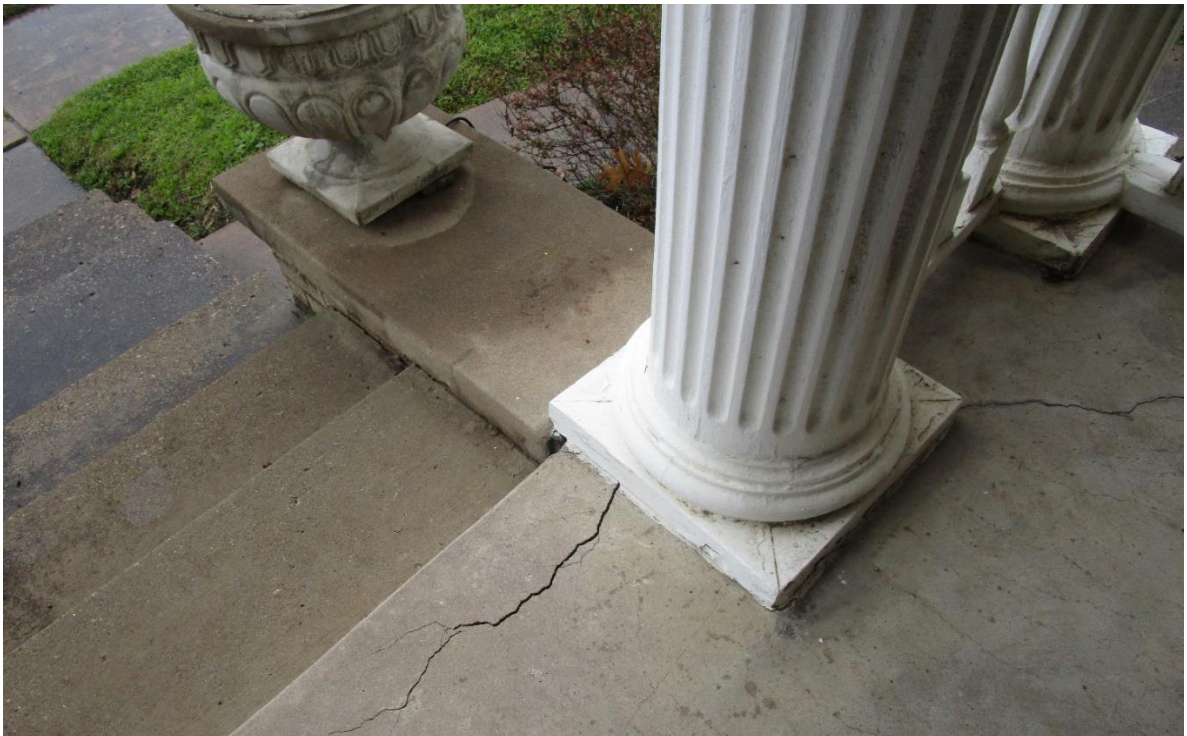
Photo #29 Damaged concrete slab at the south patio.
