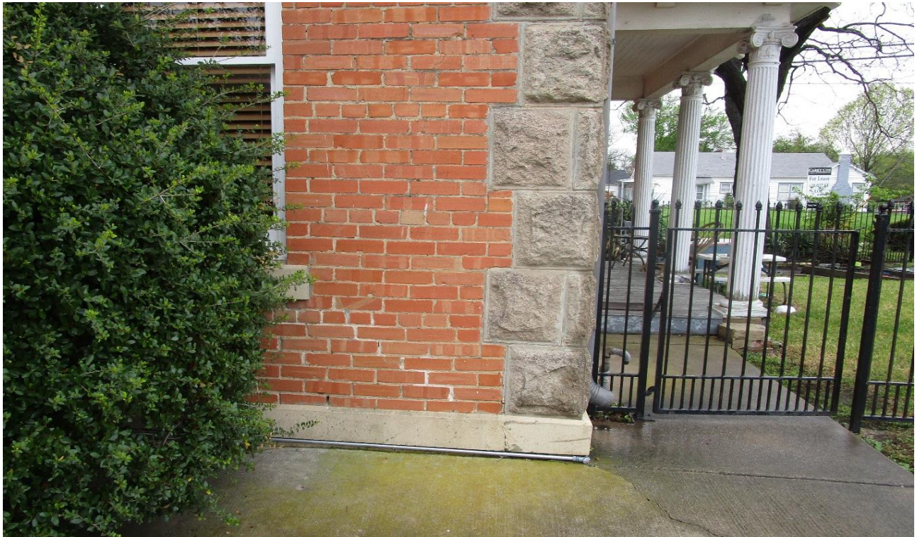
Photo #2 Northwest corner of the north side of the building. the corner of the building has experienced some foundation movement in the past.
