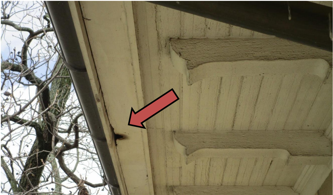
Photo #51 Arrow points to a hole in the roof soffit that is likely due to roof rats or squirrels. This hole should be filled. Note that rodents will chew thru wood to gain access to attics.
