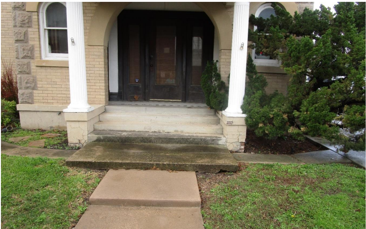
Photo #12 East entrance to the building. The stucco on the short brick walls is falling off. The steps appear to be bowing upwards in the middle, likely due to some heaving of the soil.
