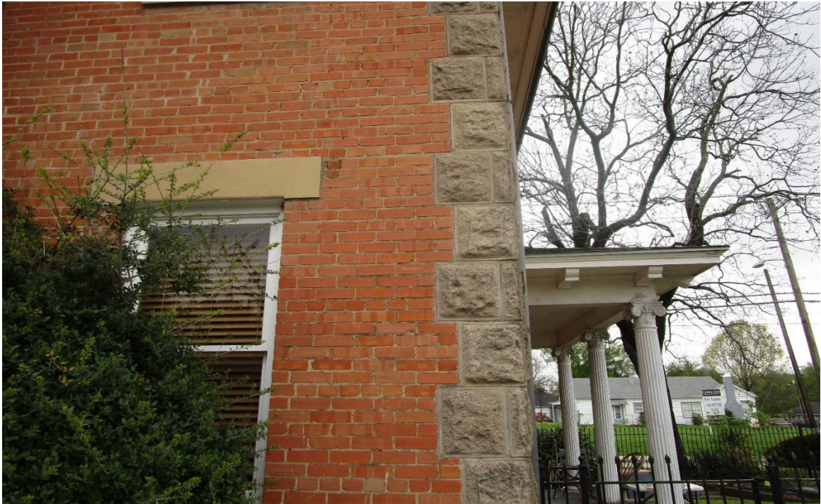
Photo #3 Some damage to the brick on the northwest corner of the building is present.
