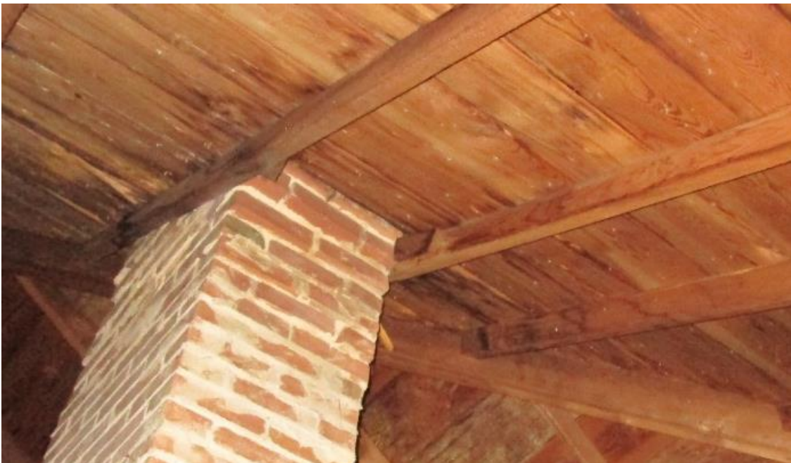
Photo #48 Close up view of the chimney – roof intersection. The decking has apparent water damage and some of it needs to be replaced.
