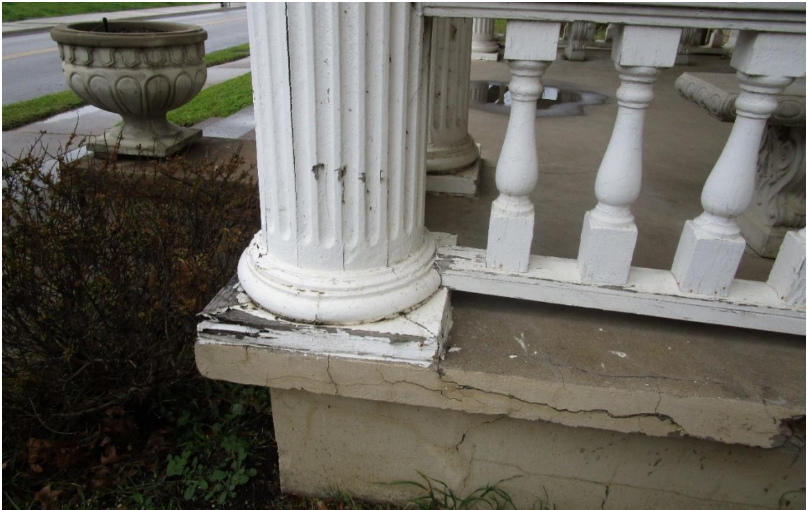
Photo #21 The wood column base has severe water damage and needs to be replaced.
