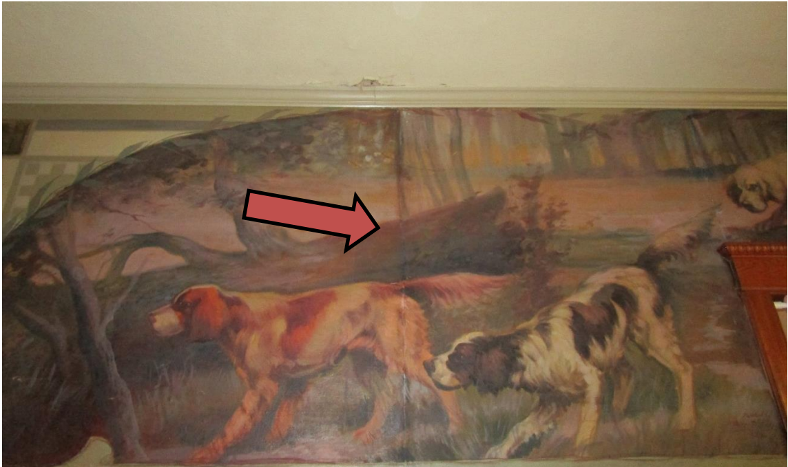
Photo #37 The arrow points to a crack in the wall mural. The crack is likely due to water from a roof leak.
