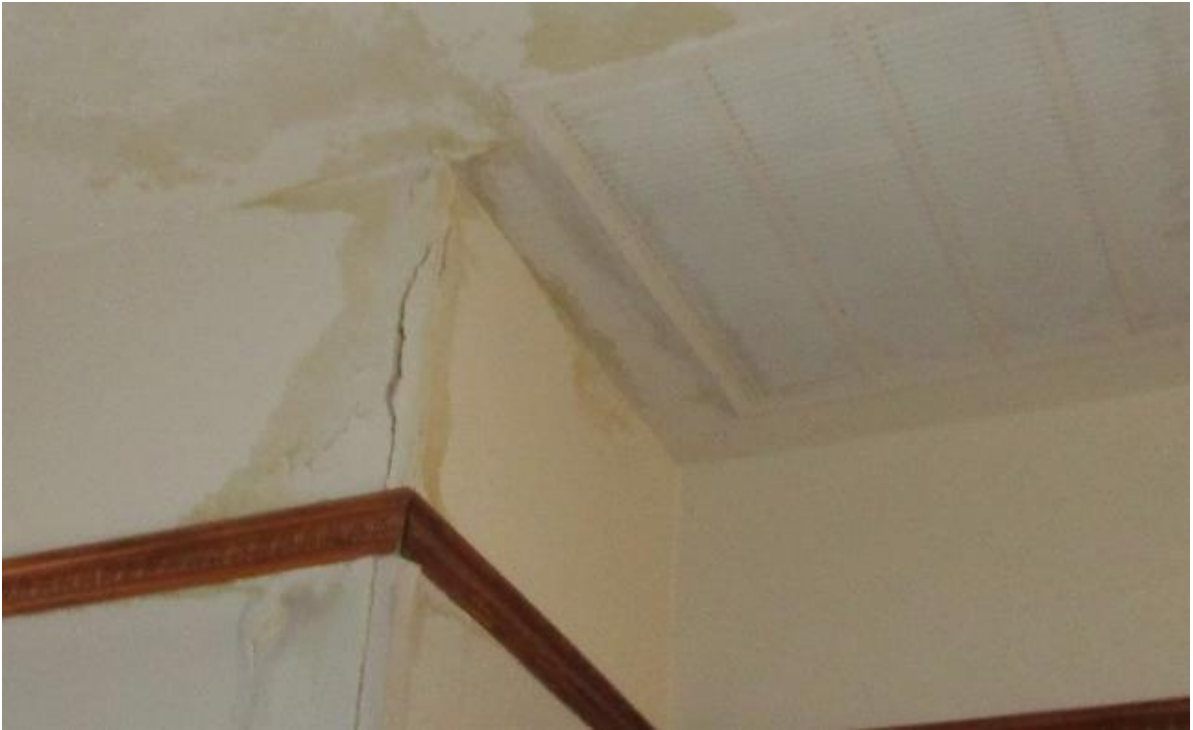
Photo #59 Close up of water damage at second floor ceiling. This is above the kitchen on the first floor where the plaster is damaged.
