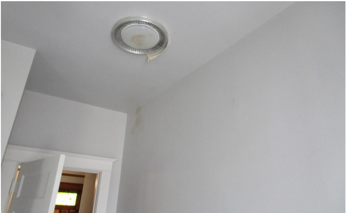
Photo #42 Some water damage to the wall near the ceiling and to the wall paper around the ceiling light.
