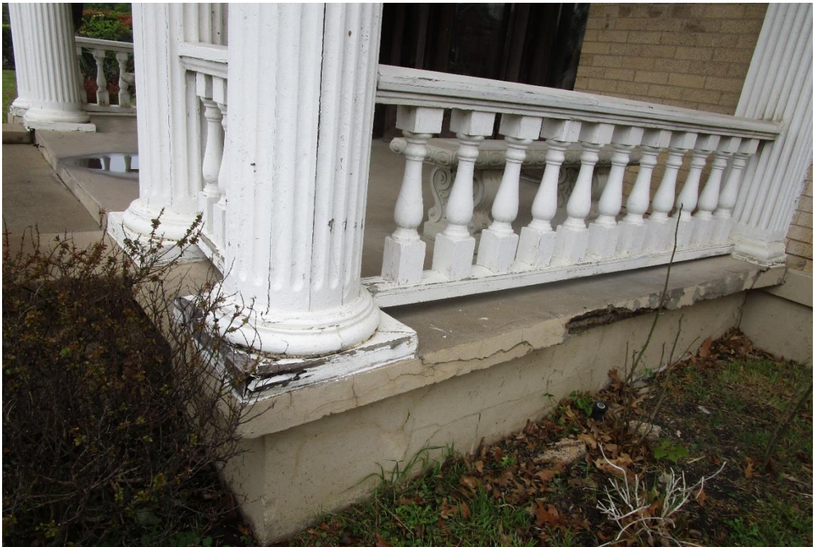
Photo #19 The column base and concrete have severe water damage.
