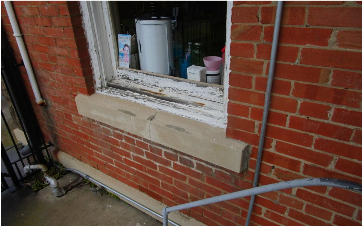
Photo #61 Windowsill on the west side of the building. The wood windowsill has severe water damage. The limestone sill has a crack in the middle.
