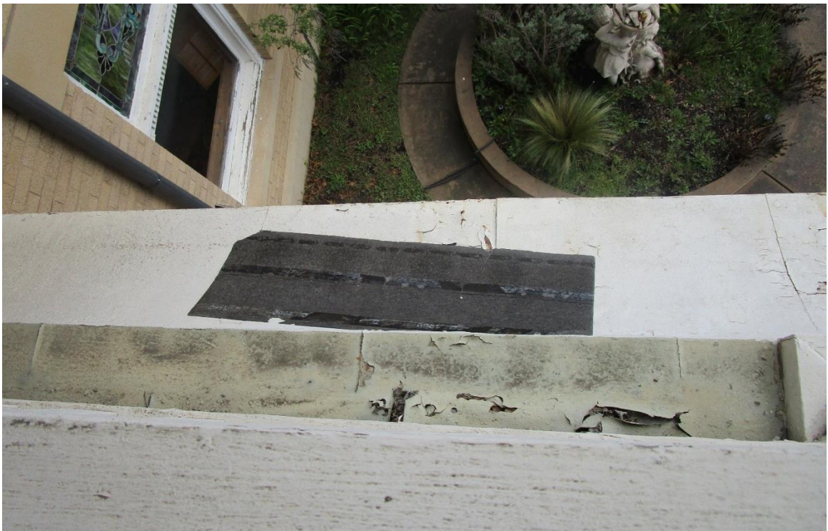
Photo #52 A roof shingle from upper roof that is laying on the east side of the lower roof for the south side entrance.
