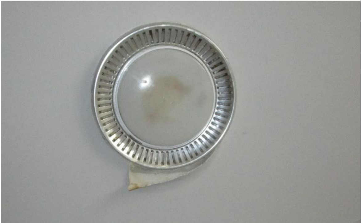
Photo #43 Close up of damaged wall paper around the ceiling light fixture. The fixture likely has water damage as well.
