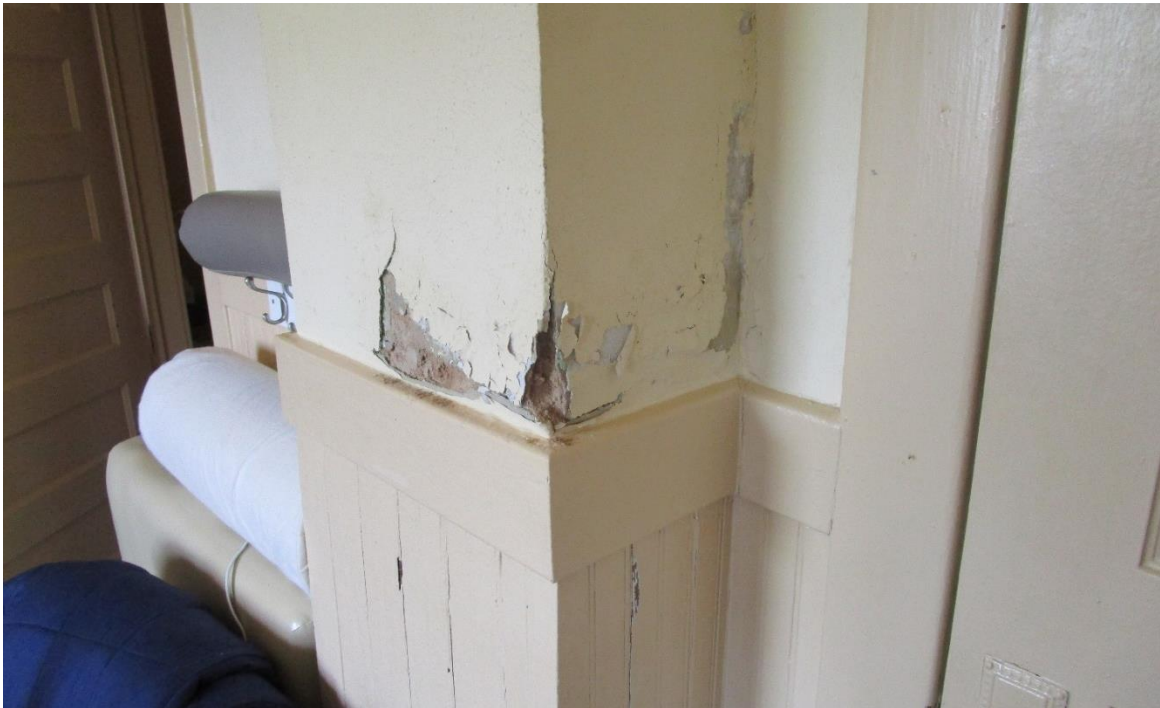
Photo #34 Another view of the damaged plaster in the kitchen.
