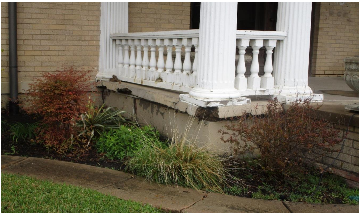
Photo #24 West side of the south covered entrance patio. This side has concrete damage and wood column base damage.
