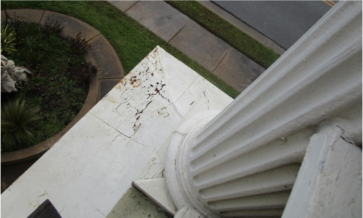
Photo #53 Crack paint on the lower roof southeast corner. It appears that the metal for the lower roof is rusting.
