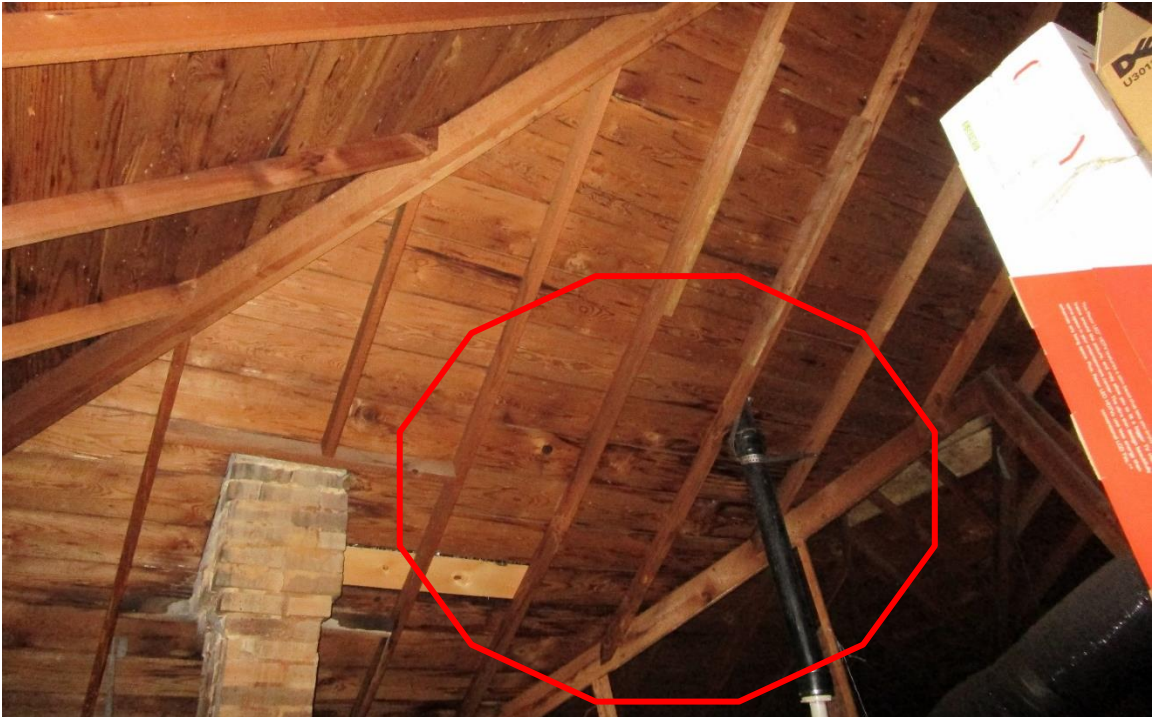
Photo #45w View of the underside of the north side of the roof. The circled area appears to have water damage. Two deck boards have been replaced. Some of the roof rafters have been repaired.
