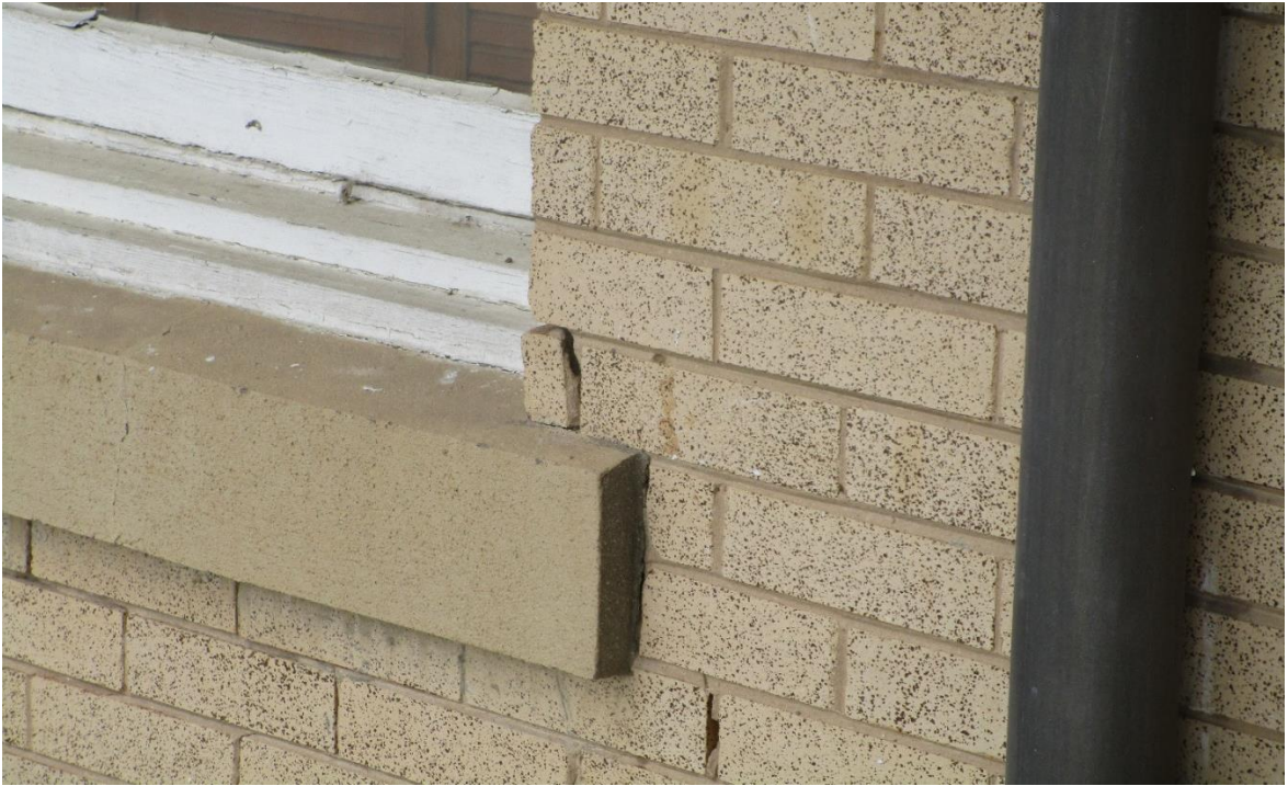
Photo #57 A small piece of brick has lost the mortar tying it to the remaining brick.
