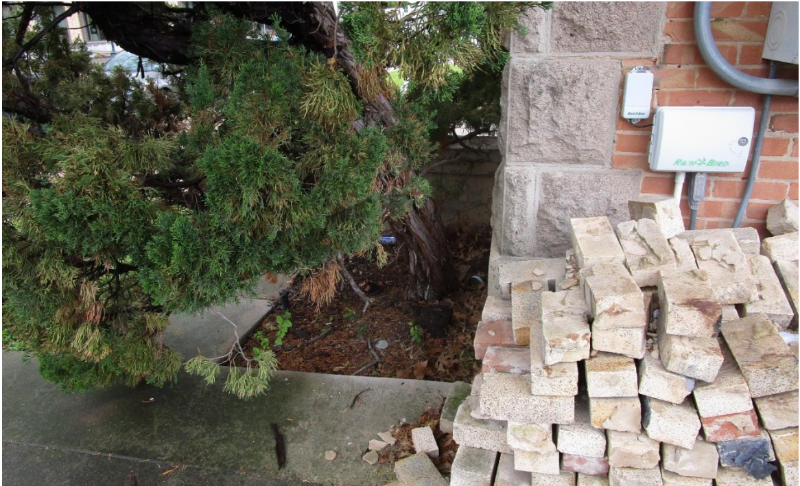
Photo #9 The trunk of the old cedar tree is within inches of the foundation. The tree should be removed.
