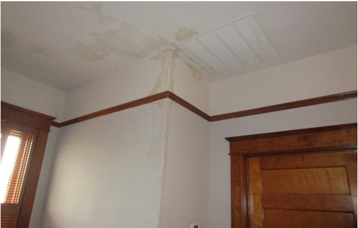
Photo #58 Water staining on the wall and ceiling in the second-floor hallway.
