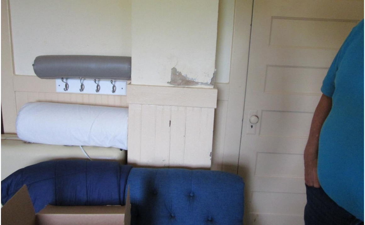
Photo #33 Damaged plaster in the kitchen. This is likely a part of the brick chimney that has water coming around the roof penetration.
