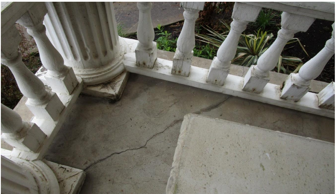
Photo #30 Damaged concrete slab at the south patio.
