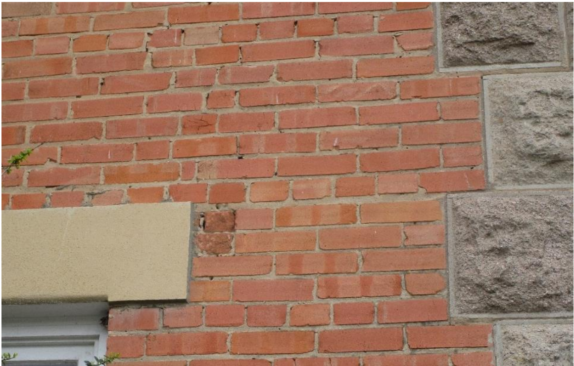
Photo #4 Close up of some of the damaged brick on the northwest corner of the building. This area needs to be tuck pointed to keep water out of the walls.
